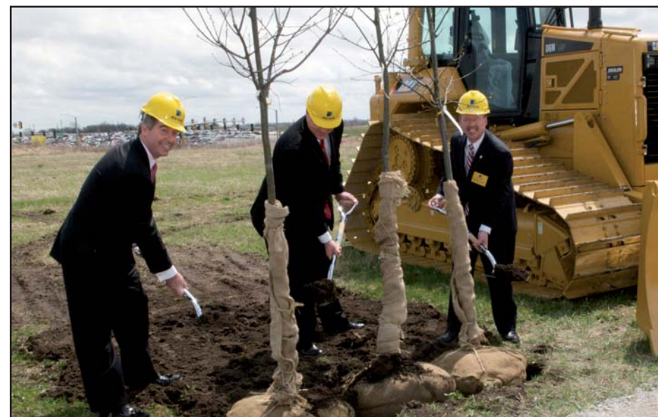
Breaking ground for Aviva's U.S. operations headquarters were (L to R) Tom Godlasky, president and CEO of Aviva USA and Aviva North America; Chet Culver, Governor of Iowa; and Steve Gaer, Mayor of West Des Moines.
